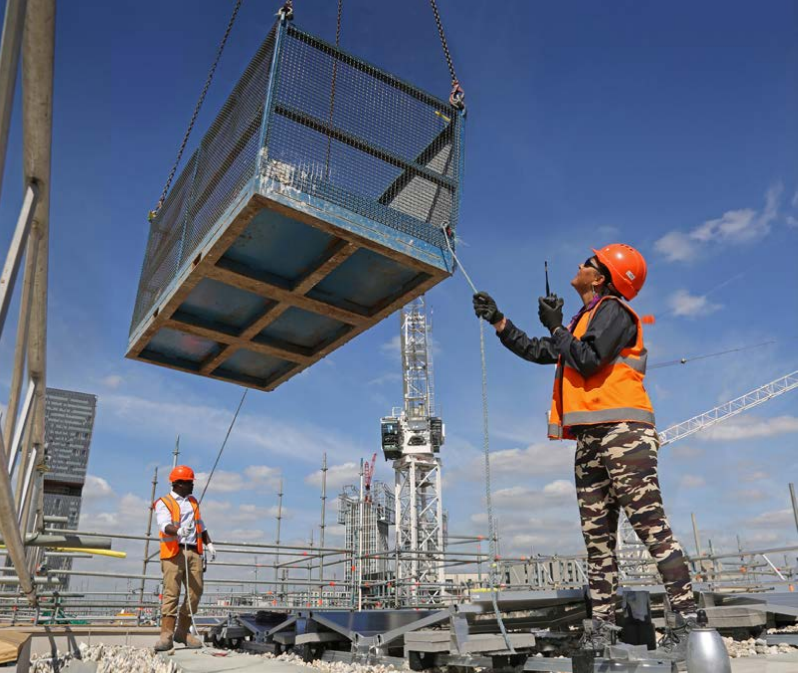
A construction worker guides an access platform as it is lifted onto the roof of a new building in London Simon Turner / Alamy
