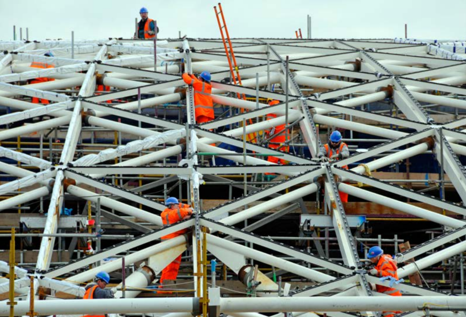
Construction workers on the new roof at Kings Cross station in London Justin Kase ztwoz / Alamy
