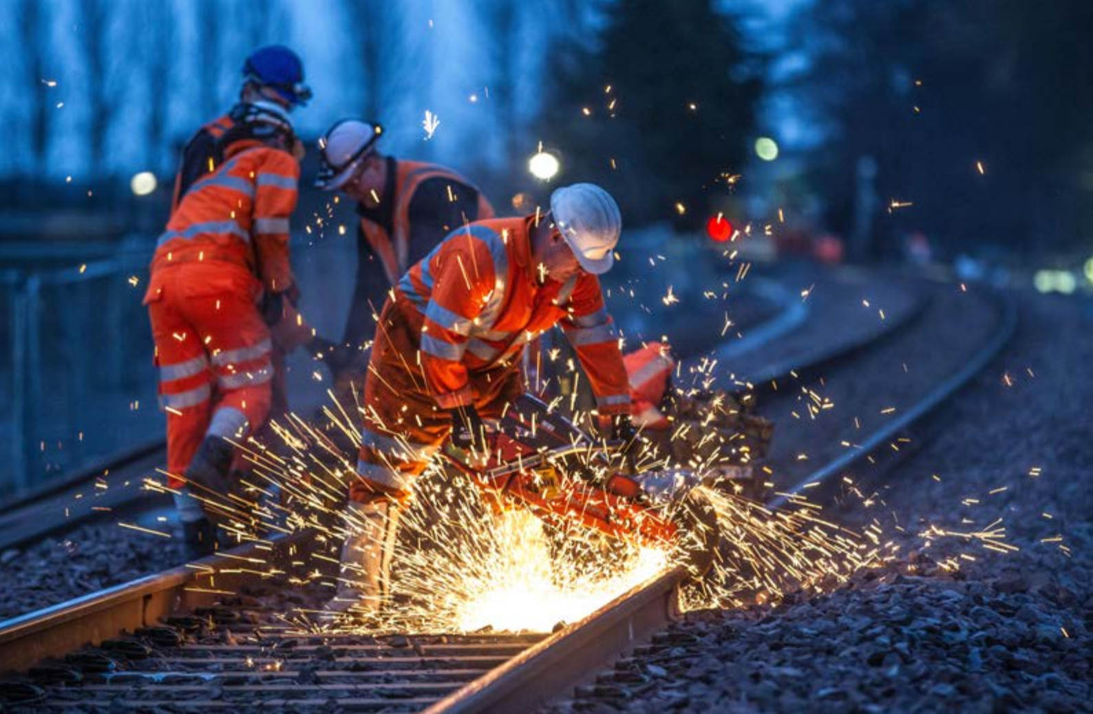
Night shift rail workers cutting and laying new tracks in Forres, Scotland Peter Devlin / Alamy
