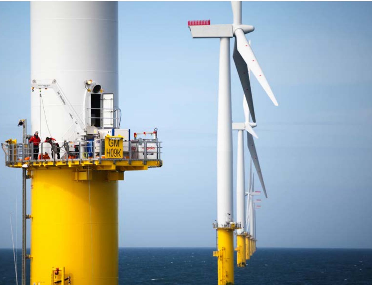
Engineers working on a turbine on the Gwynt y Mor offshore wind farm in North Wales Rob Arnold / Alamy
